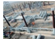
Ultra-high voltage (1,100 KV) power generation and transmission plant
