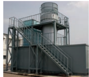
Pilot plant of non-aeration wastewater treatment system (Capacity: 30 m 3 /day) (Japan Sewage Works Agency's Research & Technology Development experimental center)
