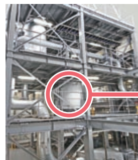
Facility for the research and development of fast reactors (sodium loop facility)
