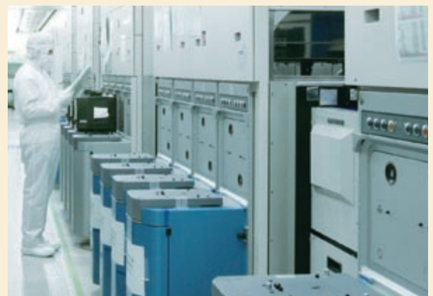
Clean rooms at the semiconductor plant use local air-conditioning systems to curb energy consumption.
