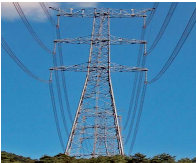
Transmission line for UHV (1,000kV) of TEPCO
