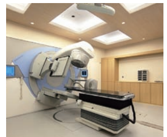
Linac system room
